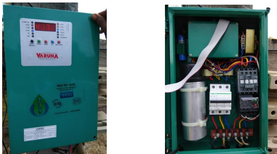
Figure 36: Smart Control Panels distributed in AgDSM in Andhra Pradesh
